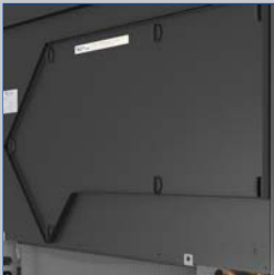
Inspection access panel for G3/F7 filter and heat recovery
