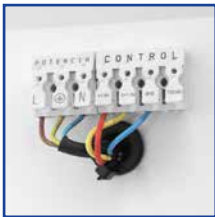
Detail from the terminals box in fancoil units
