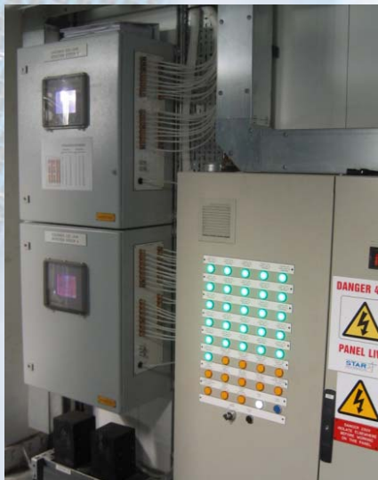
Gas Detection Panel
